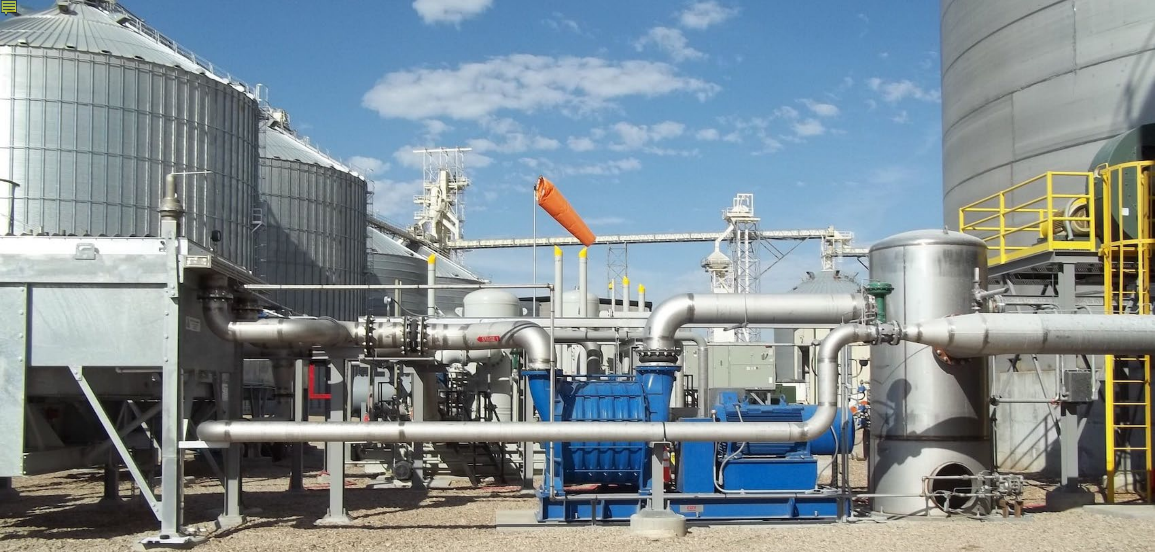
Conestoga Energy Partners Carbon Capture Project
